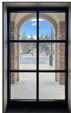
Figure 1. IGU on CU Boulder campus being evaluated for performance reduction due to degradation.
